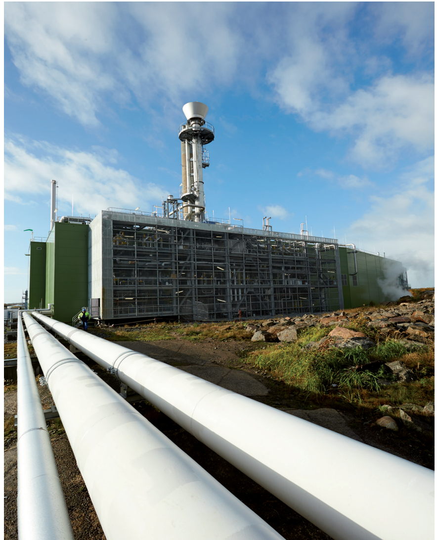
Figure 13. GoBiGas (Gothenburg Biomass Gasification) is a Göteborg Energi AB initiative and the plant is the first in the world to combine large-scale gasification with methanation. The capacity of the produced gas is to supply about 15,000 cars or 400 buses a year with biofuels.
